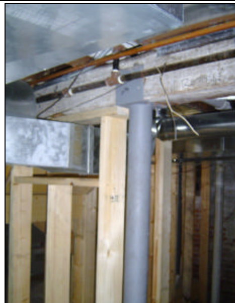
Since its construction in about 1912 the first floor had dropped nearly 2 inches. This was corrected by installing these new steel posts in the basement.
