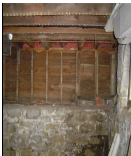
This basement view shows wooden studs resting on the original stone foundation walls.
