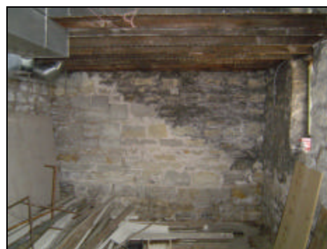
This photo was taken earlier this month. It shows the part of the basement beneath the sun porch seen in the 1940’s photo above.
