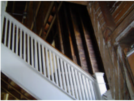
Photos taken by Fred Otto early October show the Harris home in mid-restoration. This is standing in the front hall looking from the 1st to the 2nd floor.
